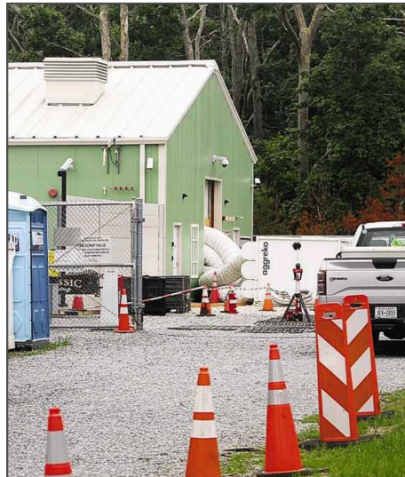
The battery storage facility substation on Cove Hollow Road in East Hampton in June 2023. A fire broke out there in May that year and the facility was back in service in July 2023.
