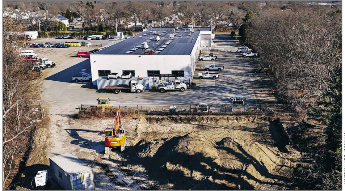
Construction has begun on a battery energy storage facility on North Ocean Avenue in Patchogue.
